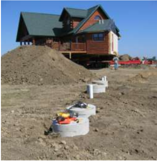
Subsurface Sewage Treatment System
