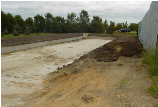
Feedlot Runoff Control Structure Completed in 2008
