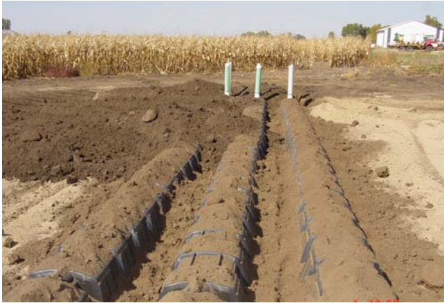
At Grade Subsurface Sewage Treatment System
